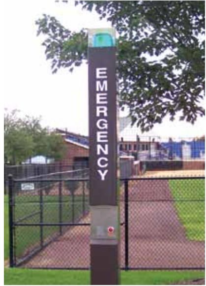
One of the many Blue Emergency Light Telephones on campus.
